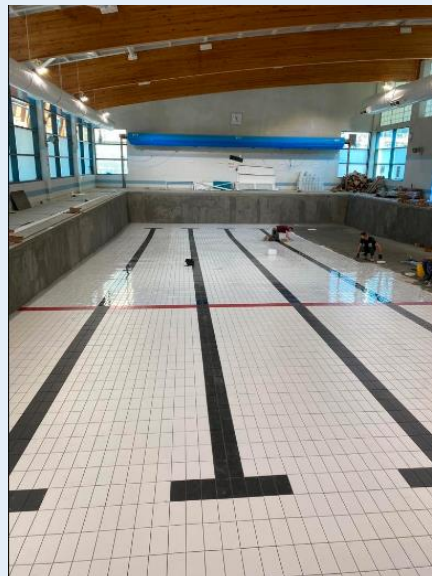
Photos: Top – View of Pool Hall, Middle – Access turnstiles, Bottom – Pool Tiling. Credit: LB Lewisham
