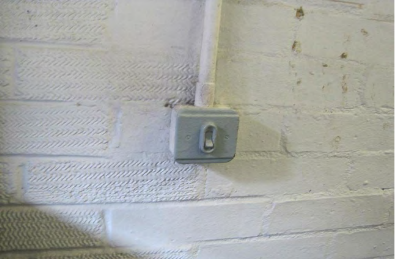
Photo No 20: Dated light fittings
