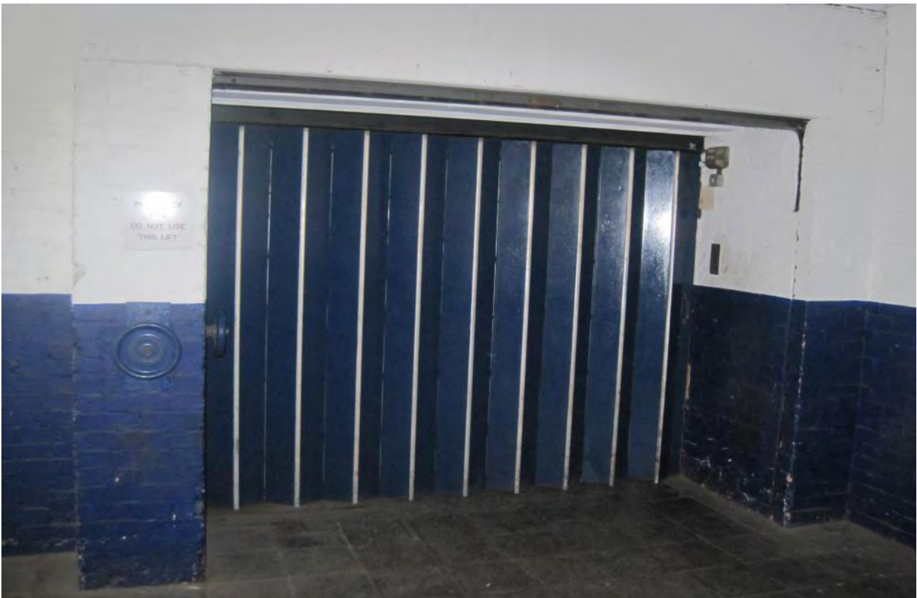
Photo No 8: Goods lift to building A
