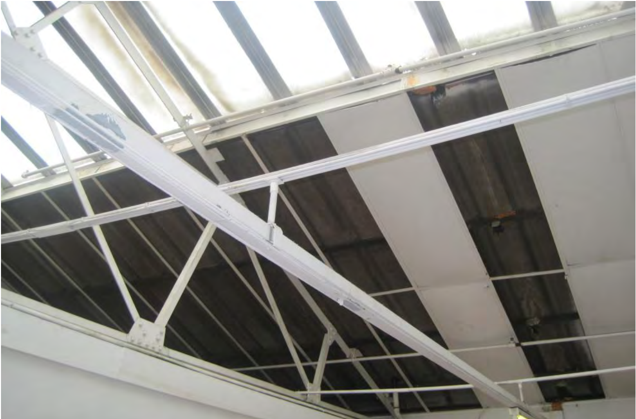
Photo No 12: Painted steel roof trusses, soffit lining boards and exposed roofing to Building A
