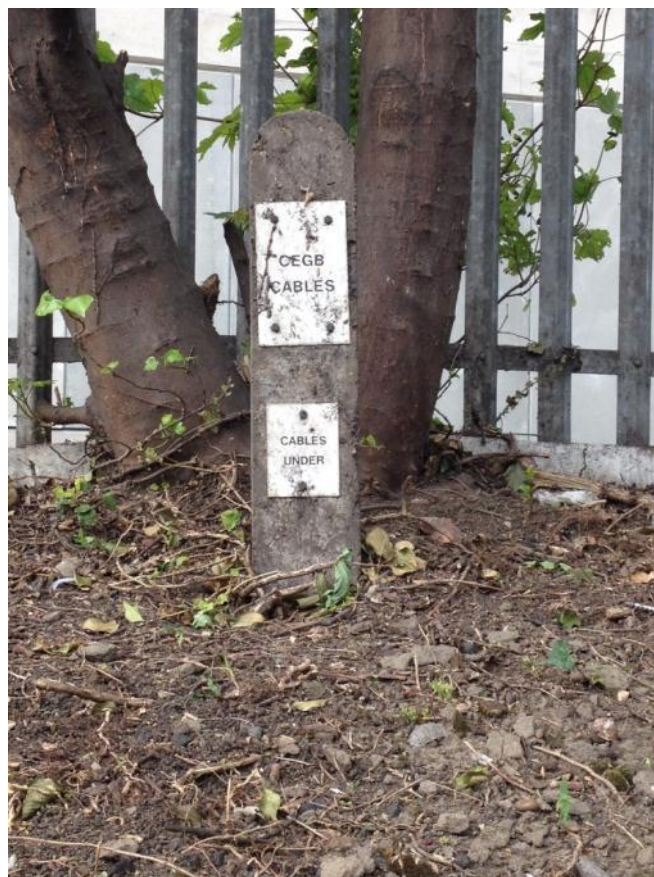
Figure 3-8: Electricity cable position markers in the verge on the south side of Surrey Canal Road
