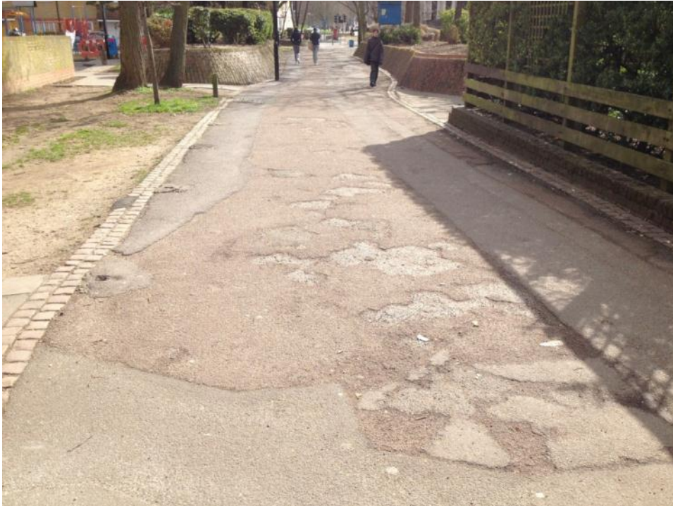
Figure 3-13: Southern end of Woodpecker Road - scarring from other utility installations
