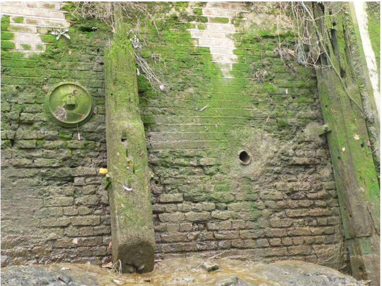
Building materials and details of the area II: Combined yellow London Stock brick and engineering brick at the railway viaduct; wire-cut brick with the old Zenith sign at the Faircharm Industrial Estate; Brick Creek wall with timber fenders
