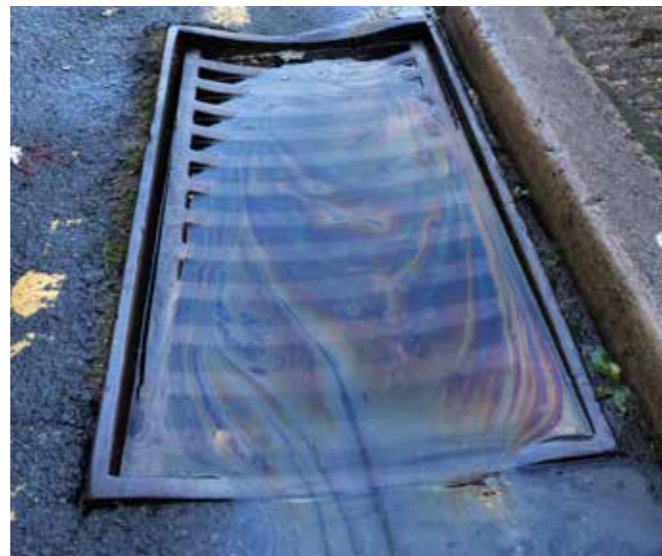
Pollution from roads and car parks is often visible - fuels, oil, heavy metals, tyre dust and silt all get washed into drainage systems.
