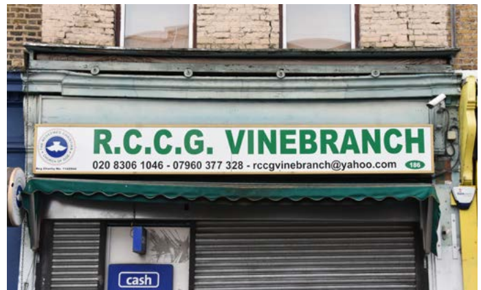
Fig. 168: Neglected historic features and roller shutters
