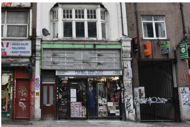
Fig. 172: Oversized signage in poor condition
