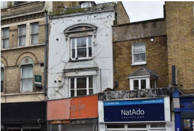
Fig. 44: Front elevations in poor condition
