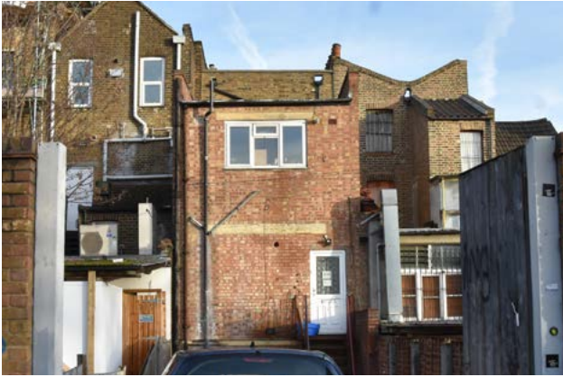
Fig. 42: Poorly detailed rear extension
